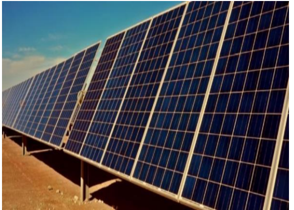
250w Solar PV panels
