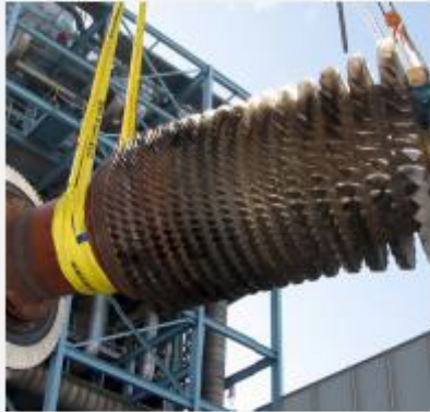
City of New Smyrna Beach, New Smyrna Beach, FL 50 MW Power Plant – Peaking Facility, 2 – Frame 5
