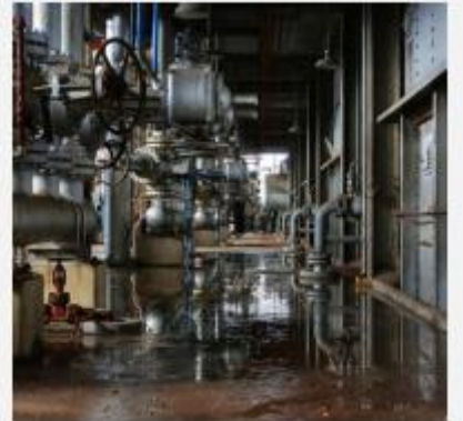
EB4104, Eastern Illinois University, Charleston, IL Fuel: Coal fired chain grate boiler
