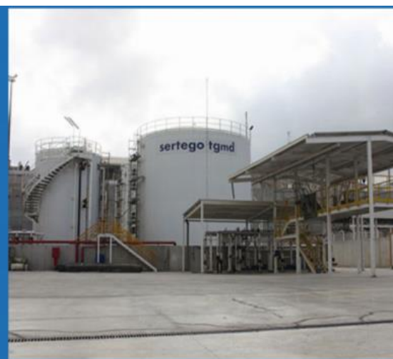
Marpol Treatment plant , SERTEGO ( TANGER), 2016
