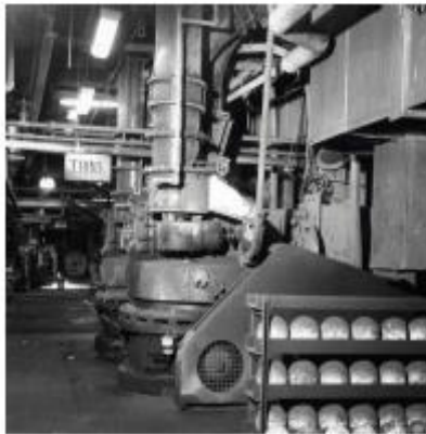
E87032 Montgomery County Incinerator Plant, Dayton, OH Fuel: Trash incinerator chain grate CE boiler
