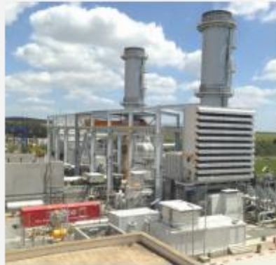
CSW Energy/ARK Energy, Bartow, FL 103 MW Combined Cycle Cogeneration Plant, 2-LM 6000 w / 25 MW STG
