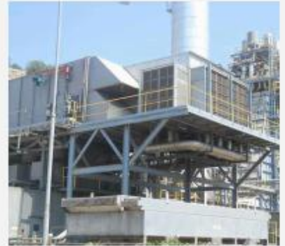
City of Calhoun, Calhoun, GA 22 MW Power Plant – Peaking Facility, 1 – LM 2500
