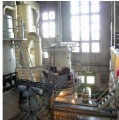
E86152 Innovest IBAE, Kuala Lumpur, Malaysia Fuel: Heavy oil (3-6% S) oil fired IBAE boiler
