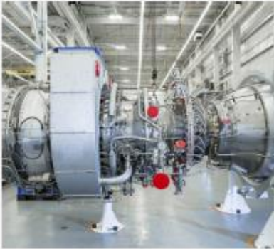
PG&E National Energy Group, Napoleon, OH 50 MW Power Plant-Peaking Facility, 2-GE Frame 5
