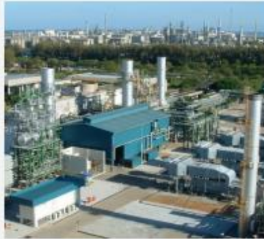
PG&E National Energy Group, Bowling Green, OH 50 MW Power Plant – Peaking Facility, 2 – GE Frame 5
