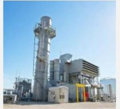
Papeles Venezolanos, Venezuela 30 MW Combined Cycle Power Plant, 1-GE Frame 5
