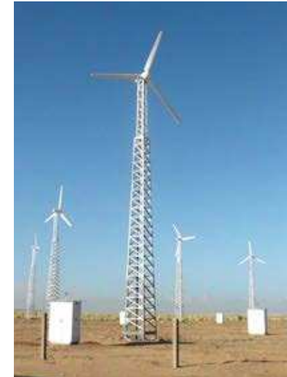
1 MW Hybrid electrification project (Wind, Solar PV & Hydropower) will provide clean and reliable energy to 165 small rural villages (selected for funding in the IRENA/ADFD Project facility)
