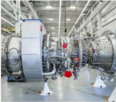
PG&E National Energy Group, Napoleon, OH 50 MW Power Plant - Peaking Facility, 2 - GE Frame 5
