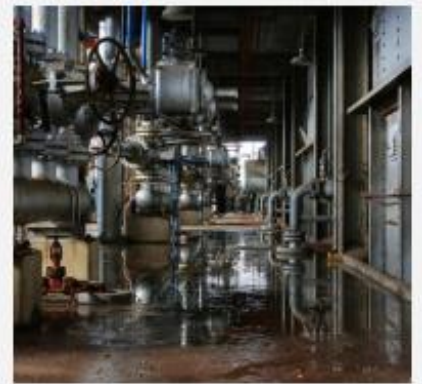
E84104, Eastern Illinois University, Charleston, IL Fuel: Coal fired chain grate boiler
