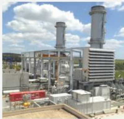
CSW Energy/ARK Energy, Bartow, FL 103 MW Combined Cycle Cogeneration Plant, 2-LM 6000 w / 25 MW STG
