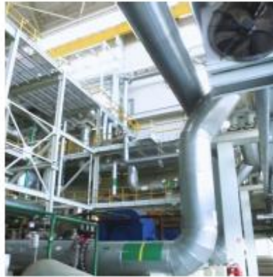
E86138 Kent State University, Kent, OH Fuel: Coal fired chain grate B&W boiler
