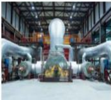
Steam power plants
