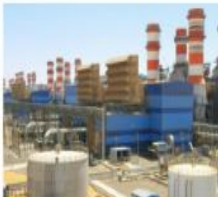
Steam turbines in CCPPs
