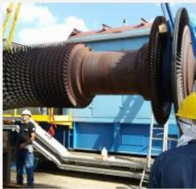
Saranac Energy Company, Inc., Plattsburg, NY 240 MW Combined Cycle Cogeneration Plant, 2-7EA, w / ACC
