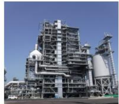
E84104, Eastern Illinois University, Charleston, IL Fuel: Coal fired chain grate boiler
