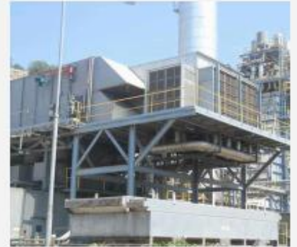
City of Calhoun, Calhoun, GA 22 MW Power Plant - Peaking Facility, 1 - LM 2500
