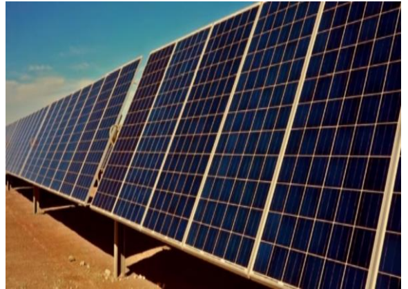
250w Solar PV panels
